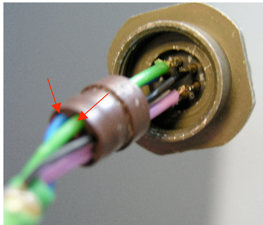
Figure 2: Miswired IQ1 connector — blue and green wires should be used with A/D pair, not A/B (JDR cable)
