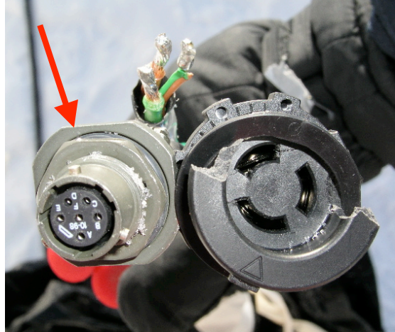
Figure 3: Wrong Connector on IQ3, JDR Cable, SJB End
